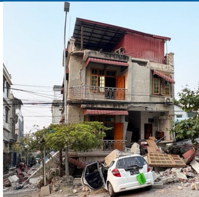
Severe damage caused to the home of Dr Khin Sandar Than, Medical Officer at The Union.
